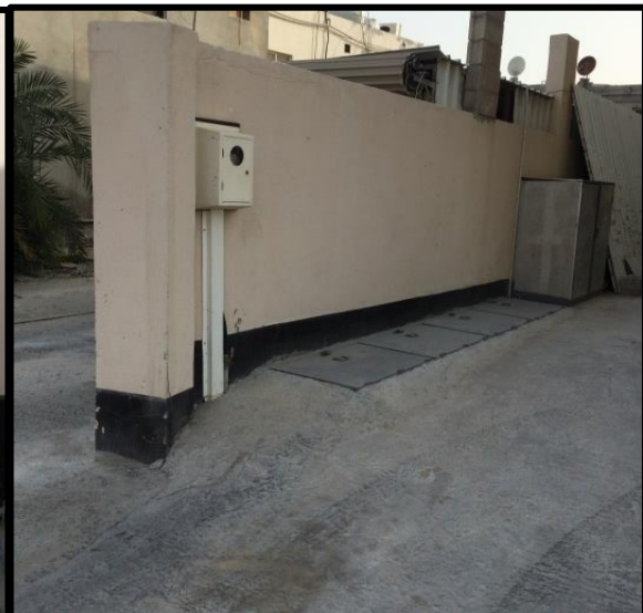
Figure 6. Wall Mounted Water Meter on Side Wall
