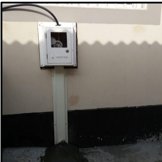
Figure 5. Wall Mounted Water Meter
